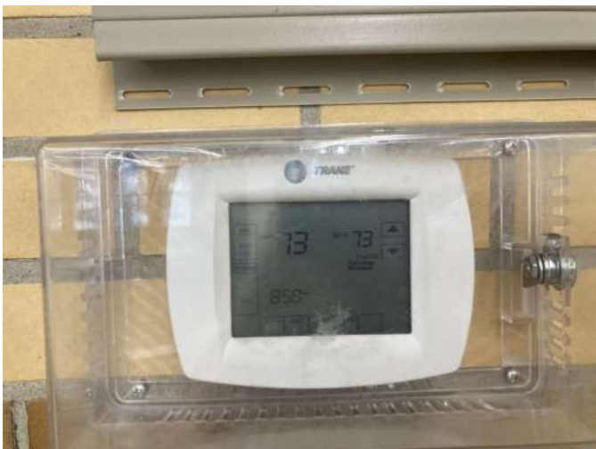
A separate heating unit and programable thermostat controls the heat in the Gesu school social hall. This eliminates heating the entire building if only this room is in use.
