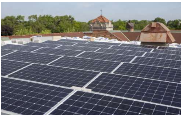
Gesu's solar array on the gymnasium roof
