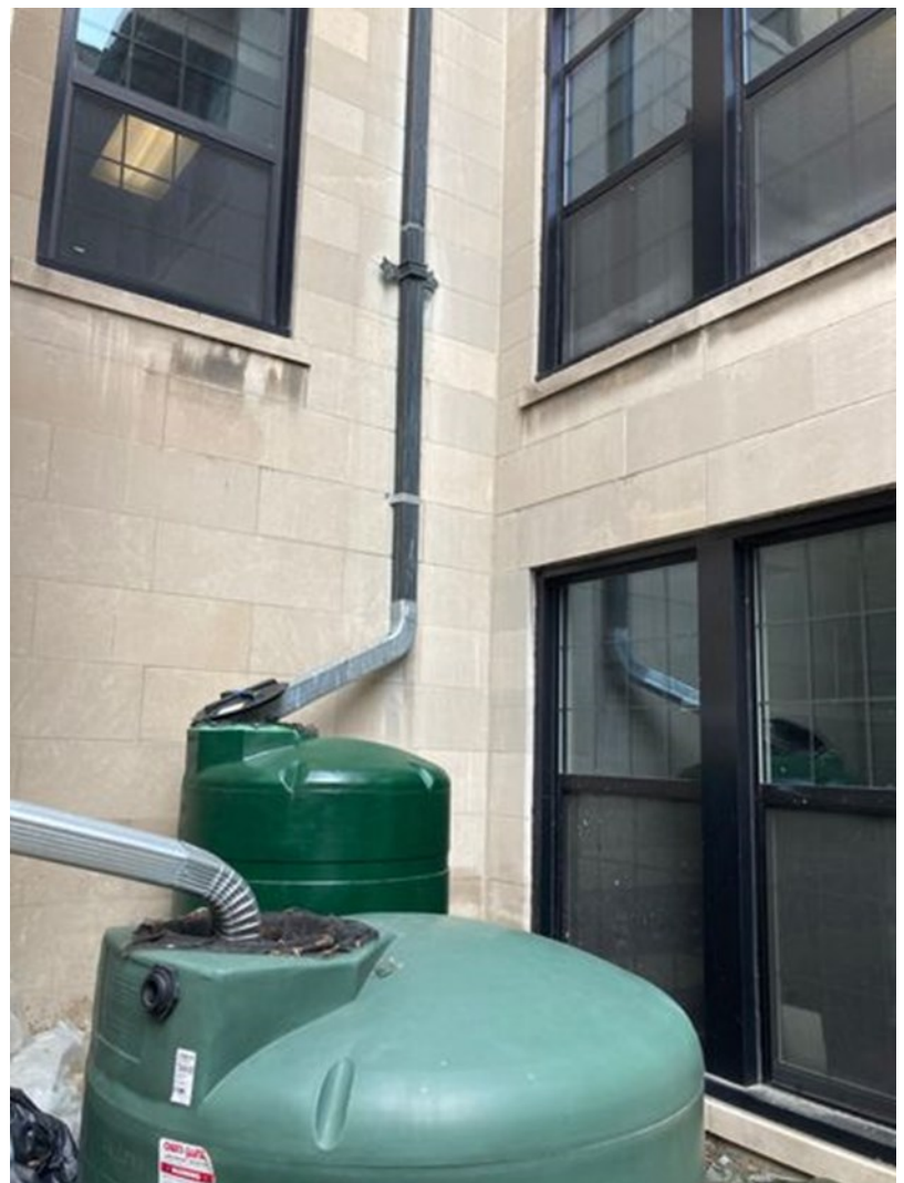
Collecting water from the roof through the downspouts
